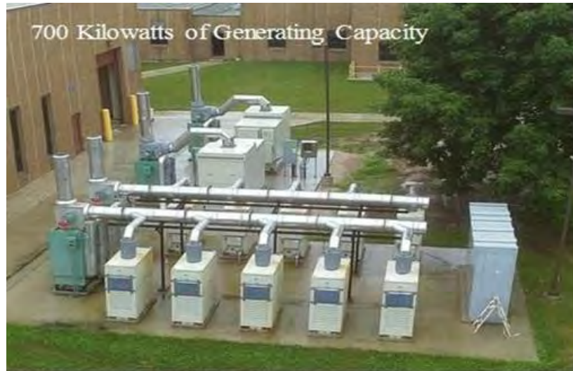
Figure 9: Microturbines at the Sheboygan WRRF
